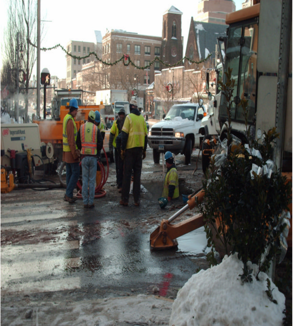
WATER MAIN BREAK MAIN STREET AND WASHINGTON STREET
